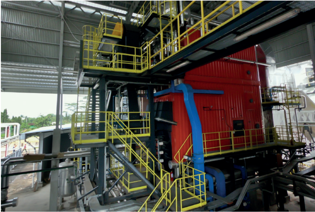
Project in Java: The engineering and construction of the 6 tph rice husk-fired water-tube steam boiler
