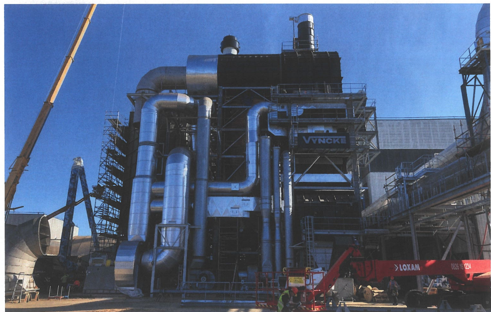
Above left: The Unilin (Panneaux de Corrèze) site at Ussel has been a focus of energy investments involving Vyncke Above right: Vyncke installation at Swiss Krono's Sully-sur-Loire plant
